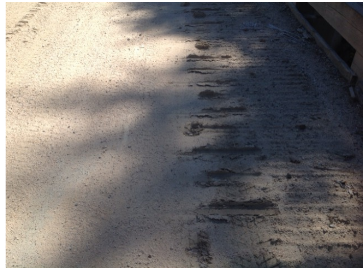
tracked machines recently walked across structure
