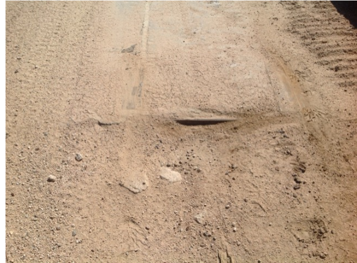
slab damage and rebar exposed
